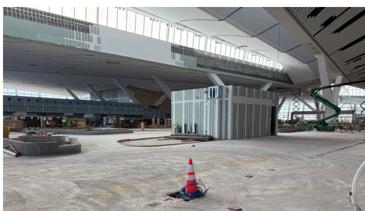
Radiant Floor Heating System Installed
