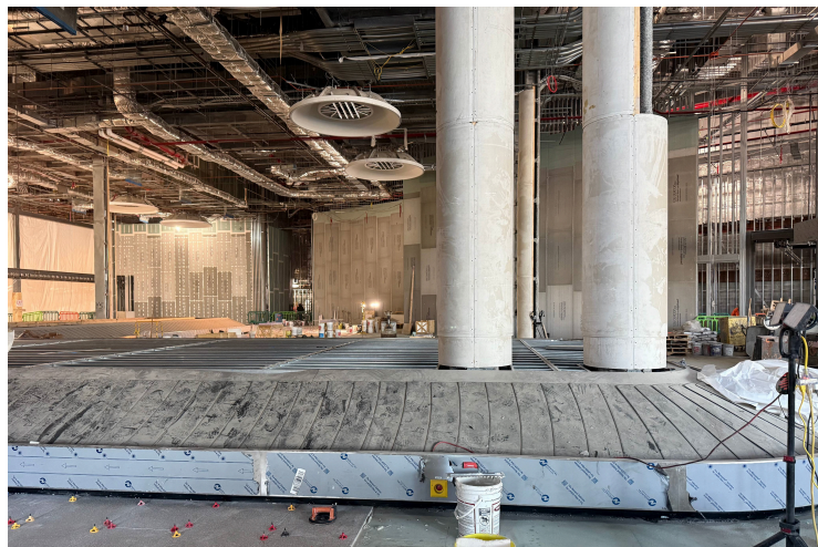
Public-Facing Baggage Handling System
